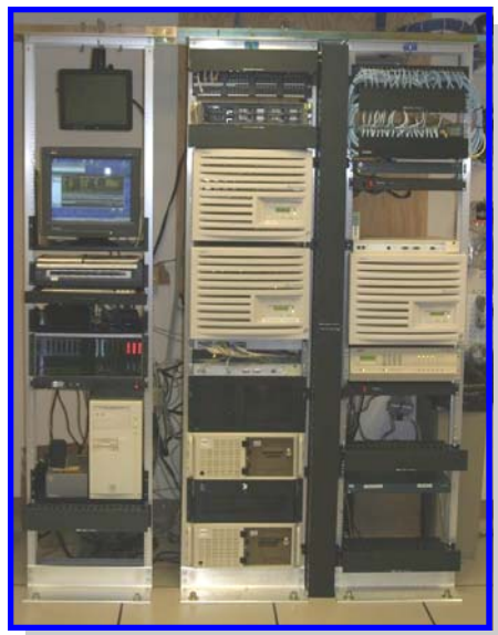
Server Rack in Computer Room
