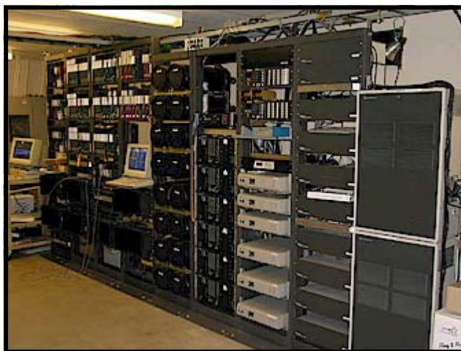
Radio Equipment Room
