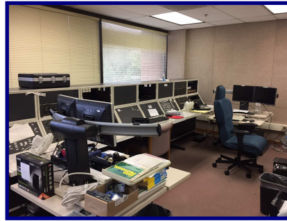
Watsonville Alternate Site before the redesign and installation of the new radio console system.
