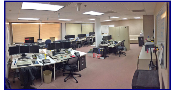
Watsonville Alternate Site after the redesign and installation of the new radio console system.
