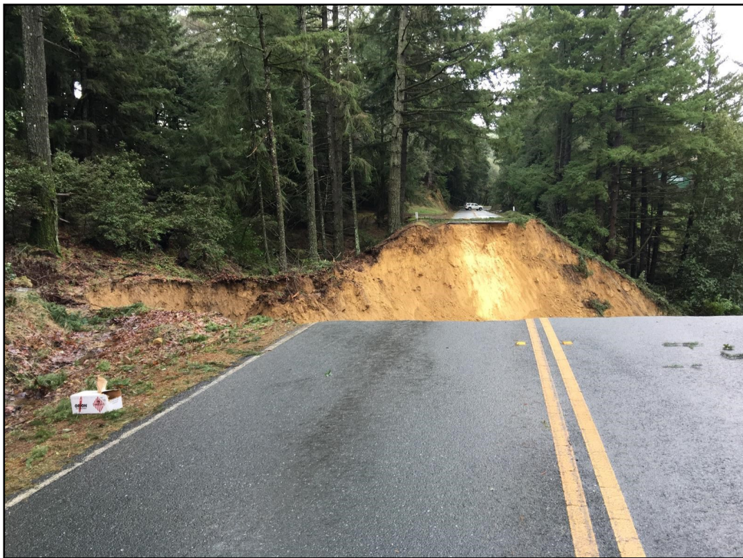
State Highway 35 following the 2017 winter storms
